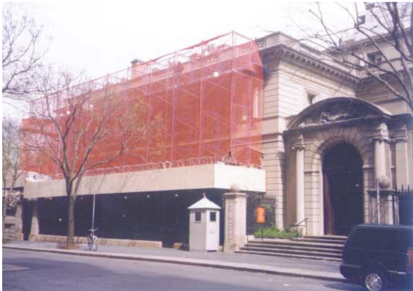
Last spring, scaffolding went up while stonework restoration was completed on the building's entire façade. Further work on the walls surrounding the Fifth Avenue and Seventieth Street gardens will continue through summer 2001.
