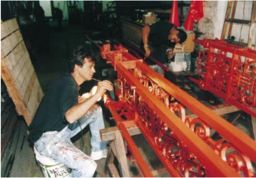
The 2001 restoration project included repairing the wrought-iron fence that surrounds the Fifth Avenue Garden. After being stripped down to bare metal, the fence was hand-painted with a rust-inhibiting primer before two coats of black paint were applied.
