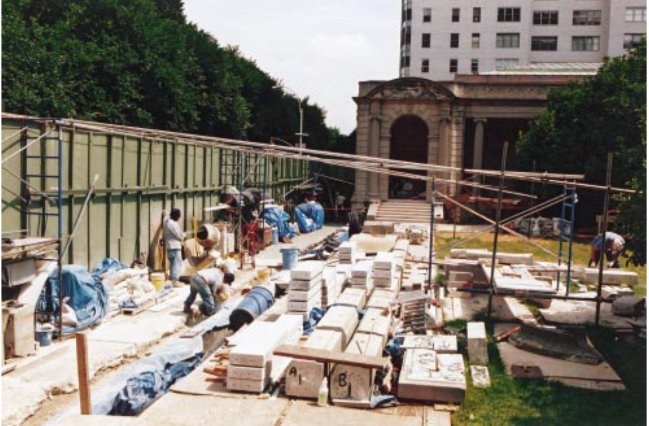
Workers in the Fifth Avenue Garden rebuild the stone wall and stairway after repairing deterioration caused by years of water damage. Whenever possible, original stones were recarved to remove damaged surface areas, then rebuilt into the repaired structures.
